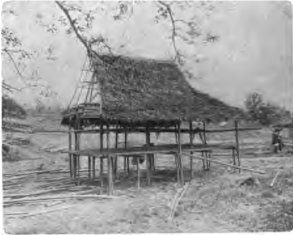
FIG. 4.—Moro house (Philippines) under construction at the St. Louis Exposition. Note the forks and rafters.
